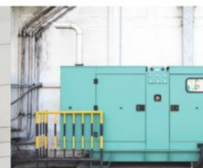
POWER BACKUP (DG)
